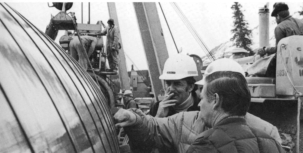
William Wilson ( right, front ), director of SDC's 80-person staff on the Alaska Pipeline Program, monitors construction of the 800-mile oil pipeline with team members.
